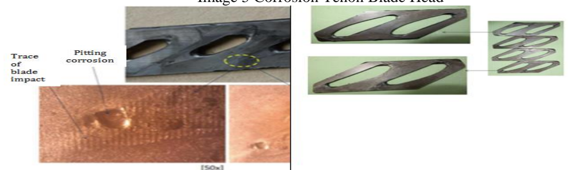
Figure 6 corrosion pitting on the surface of the bottom shroud
