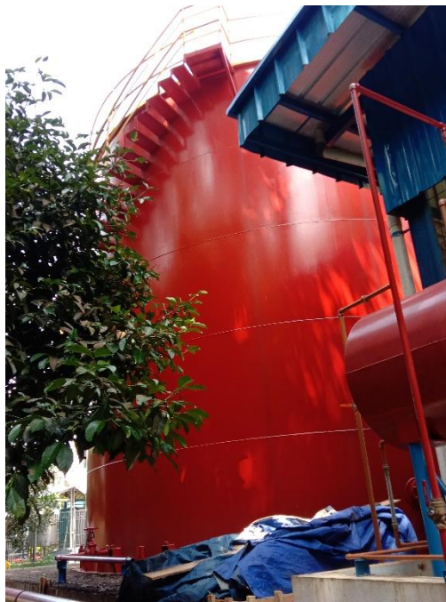
Gambar 4.3 Dokumentasi Water Storage Tank
