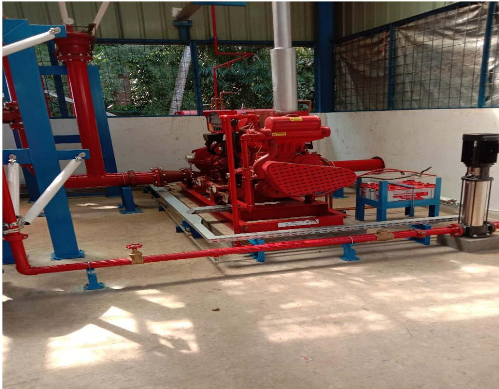
Gambar 4.2 Dokumentasi Diesel Pump
