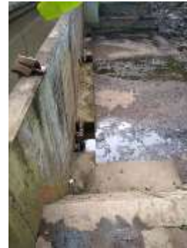
Gambar 4. 7 Valve Unit Prasedimentasi
