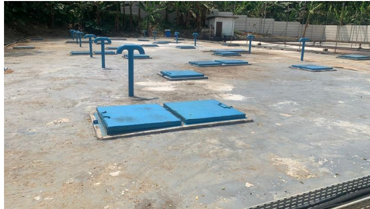
Gambar 4. 14 Kolam Anaerobik Baffled Reactor (ABR)
