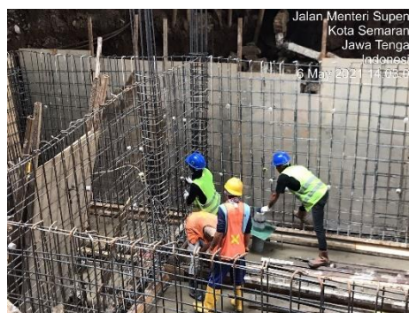
Gambar 5. 2 Ground Water Tank Air PDAM
