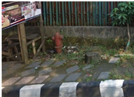
Gambar 3. 10 Fire Hydrant Jl.Cisarua
