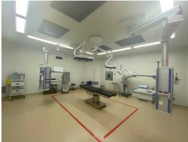
Gambar 2.6 Ruang Operasi RSBP
