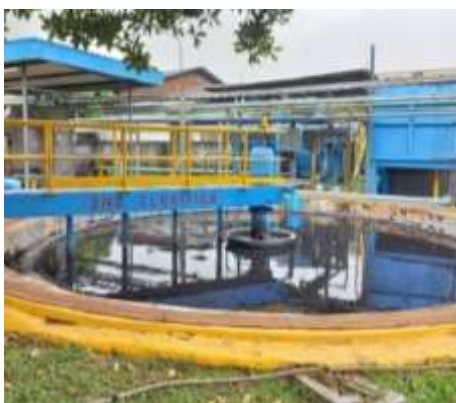
Gambar 5. 43 Bak Clarifier II IPAL PT X
