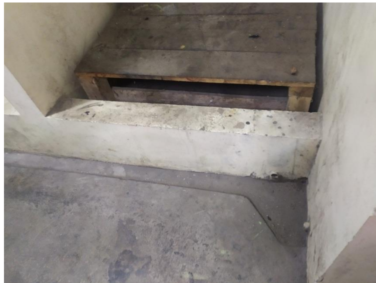
Gambar 4. 8 Saluran Drainase di TPS Limbah B3 PT Nikkatsu Electric Works
