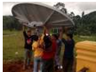
Fig 1. Broadband Internet Access Installation Source: Cikadu Village
